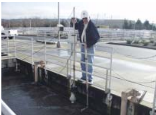
Jim Pitts, Senior Process Analyst, demonstrates how the in situ OptiQuant SVI Sludge Volume and SVI Analyzer sampling vessel is installed at the Renton plant. In his left hand is the second OptiQuant probe for suspended solids measurement.
